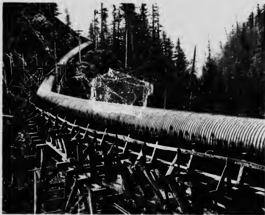
Granby Consolidated Mining, Smelting and Power Company Limited. 72 Inch Wood Stave Pipe Line on Trestle.
